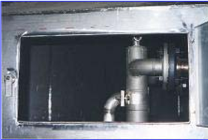
JET in operation in a production plant
